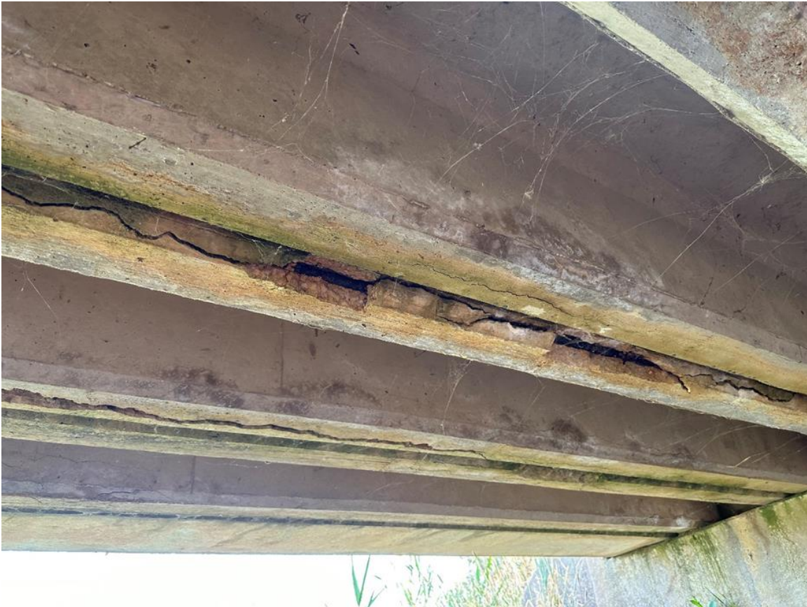
Image 3: Bridge 7 Cracking of the U-Slab beams from the underside of bridge
