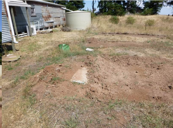
PH21. Existing wastewater treatment system servicing restaurant / function centre building
