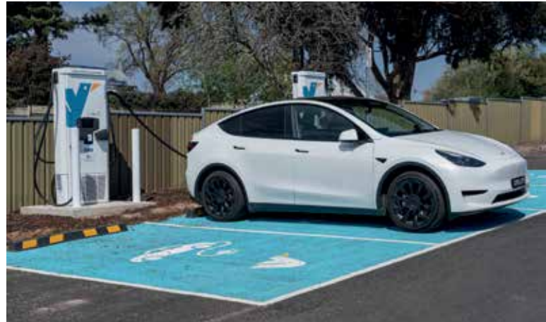
The new EV charging station joins a recently installed facility in Amphitheatre as part of the Pyrenees charging network.
