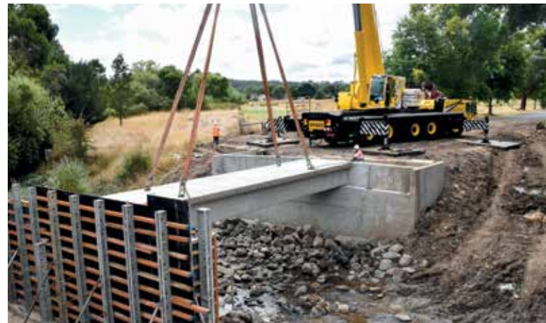
Council's Bridge Renewal Program has facilitated the replacement of several bridges, enhancing safety for all travellers.
